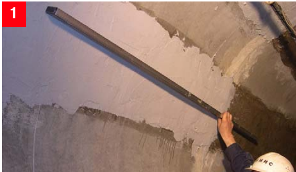
1 Areas of uneven concrete substrate had to be reprofiled with Sikadur®-41 epoxy mortar
