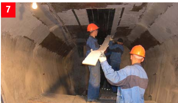
7 Installation of the Sika® CarboDur® CFRP Plates. Pressed into position by roller
